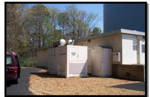
Sound attenuating Generator Enclosures were provided at two stations.
